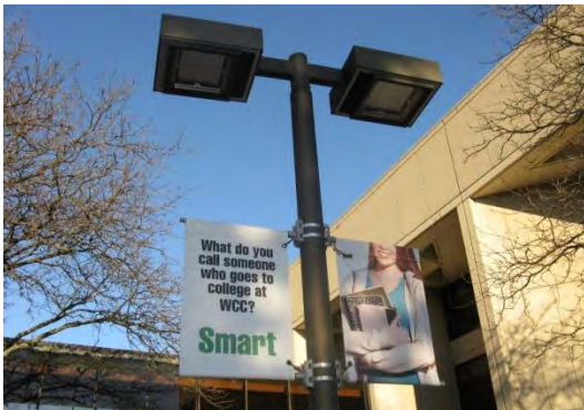
Campus walkway lighting has been converted to energy efficient LED fixtures.
