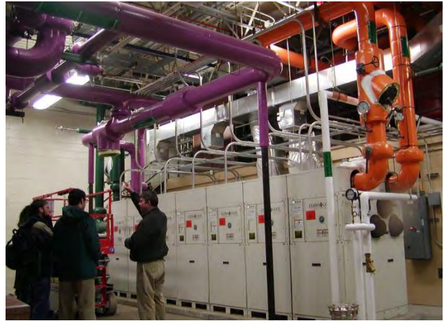
Energy Manager Bill Ghrist explains the geothermal system that heats and cools Occupational Education building. The project is expected to be LEED Gold.
