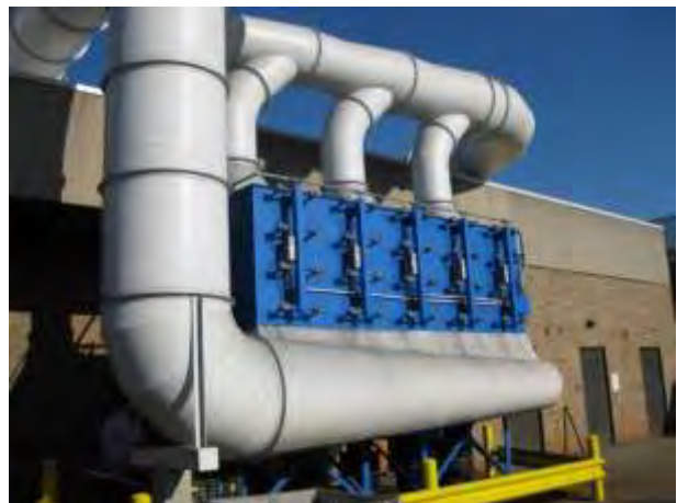
Figure 34: Welding shop exhaust system
