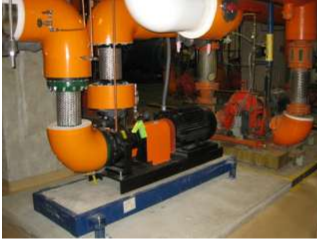
Figure 20: High temperature hot water pumps, replacement on left and original on right
