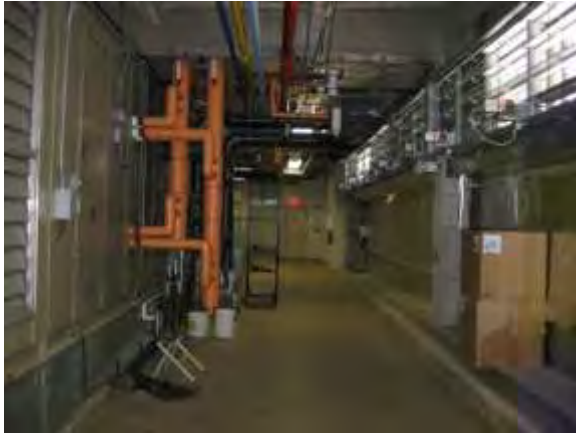
Figure 23: Air handling unit with outside air dampers
