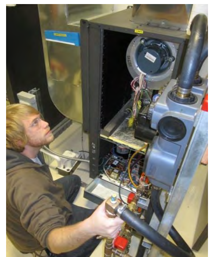
HVAC students learn to install and troubleshoot heat pumps in the HVAC lab, which are tied to the geothermal field used to heat & cool the building.
