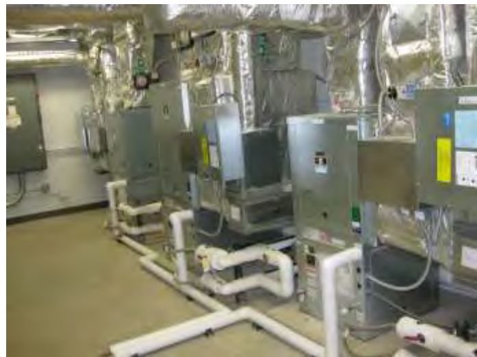
Figure 13: Mechanical heat pump systems
