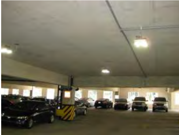
Figure 10: Parking structure LED lighting
