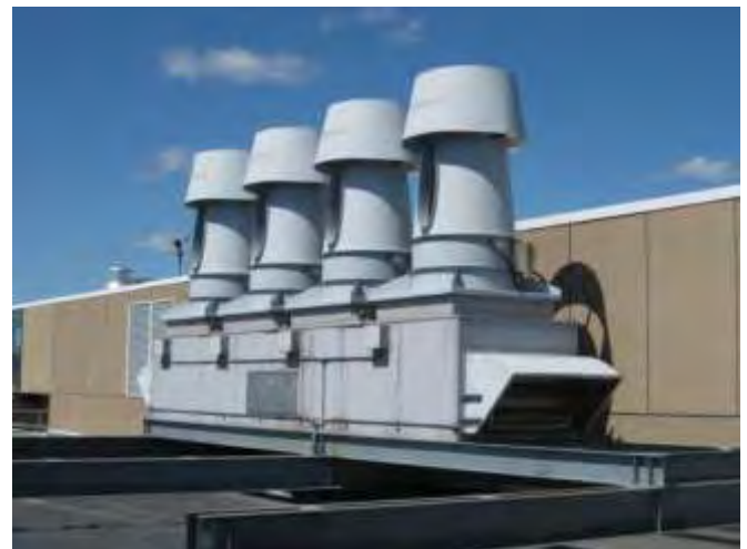
Figure 15: Laboratory exhaust fans
