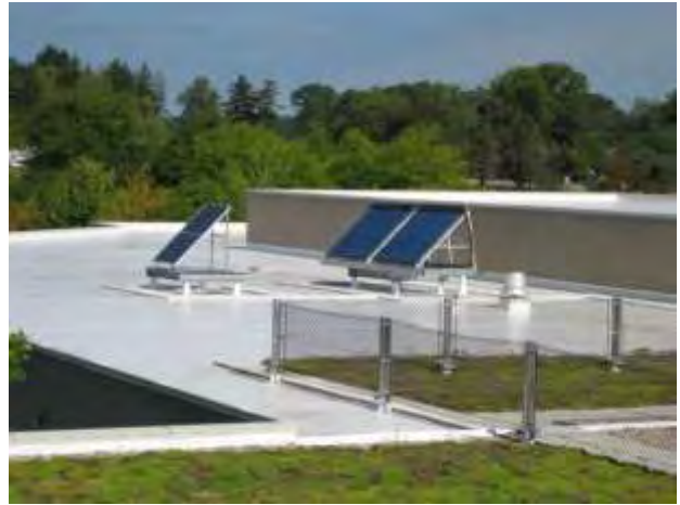
Figure 30: Roof view with solar PV and thermal arrays
