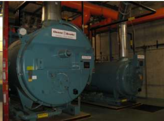
Figure 19: Main boiler and summer boiler
