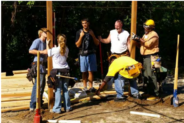
WCC construction students put beams in place to support the vegetative “green roof” over the adobe pizza oven at the Growing Hope Center in Ypsilanti.
