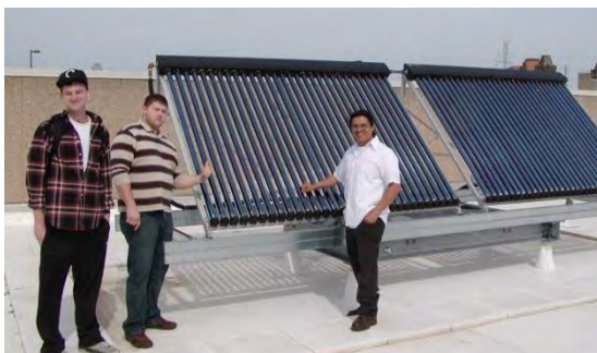
Renewable Energy students inspect the evacuated tube solar hot water collectors at the Occupational Education building.
