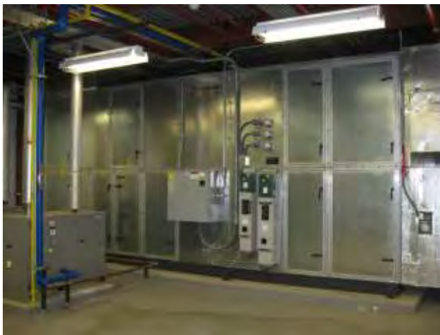
Figure 40: Energy recovery unit
